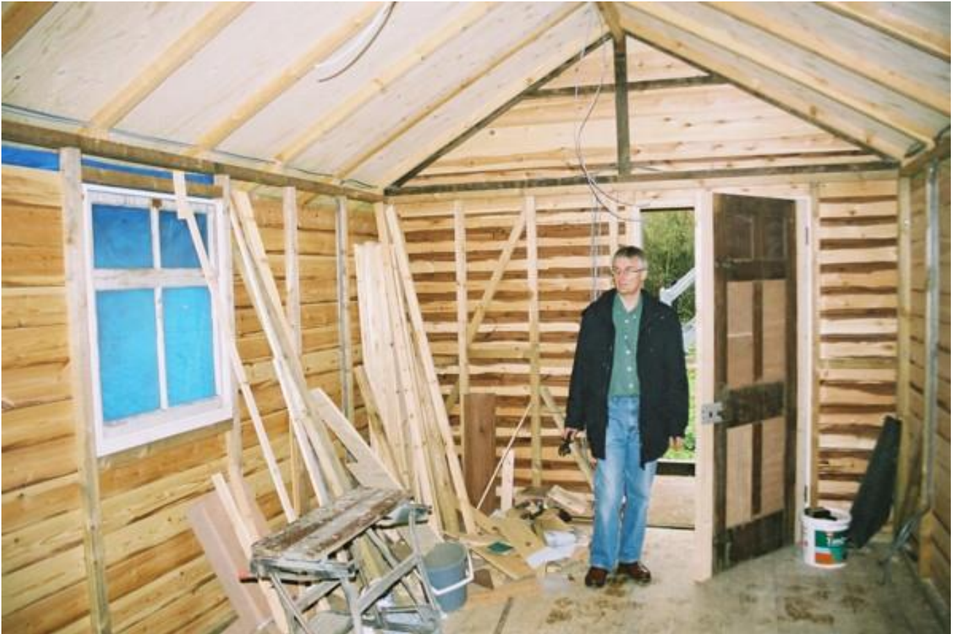
Garth Long inspects the inside of the pavilion where the displays will stand
