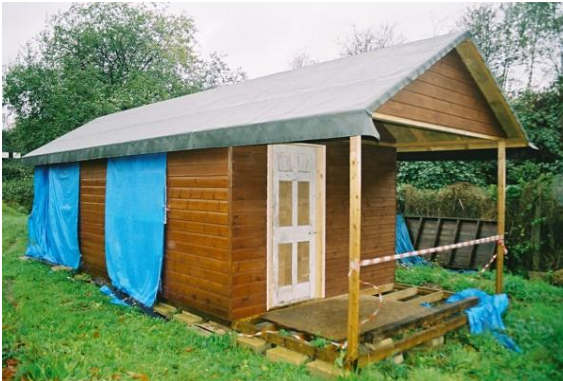
Exterior of Pavilion: Shutters still to be fitted to windows, and flooring needed
