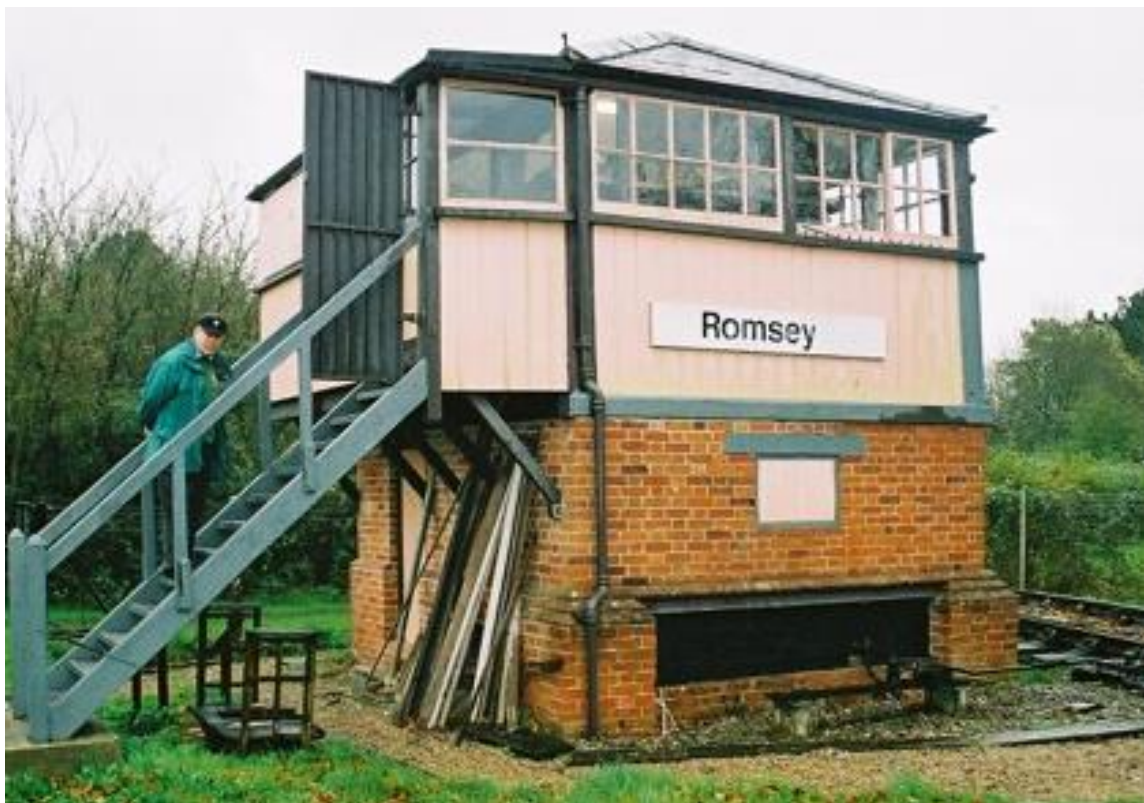
Colin Meheux tests out the rotting steps!
